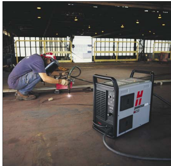
A shipyard employee in North Kingstown, Rhode Island uses plasma on a track burner
